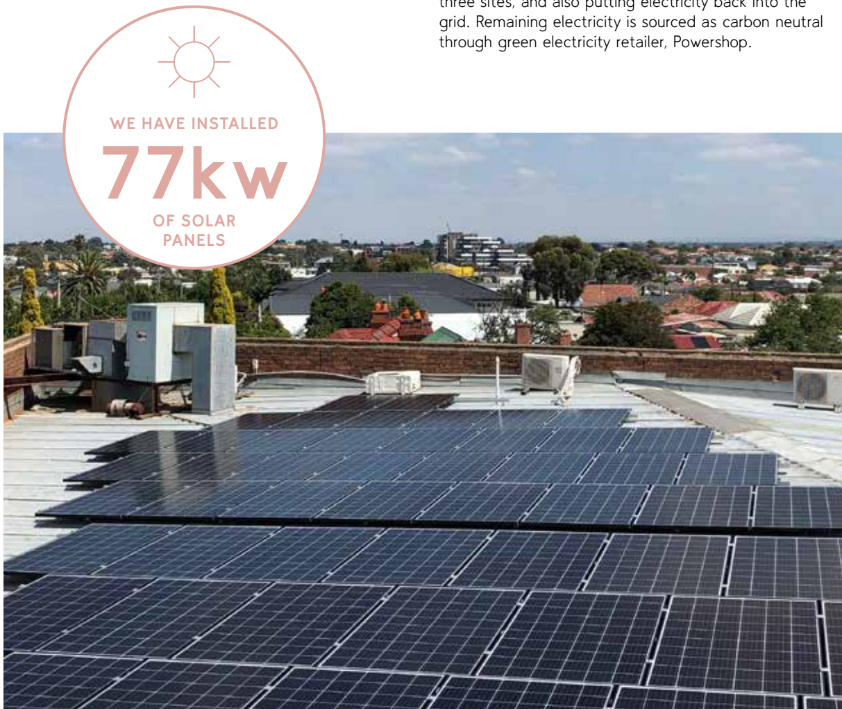
IMAGE: Newly installed solar panels at our Preston location
